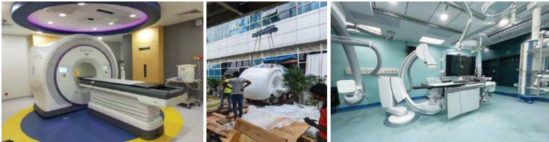
Linear Accelerator in Hospital Kuala Lumpur
