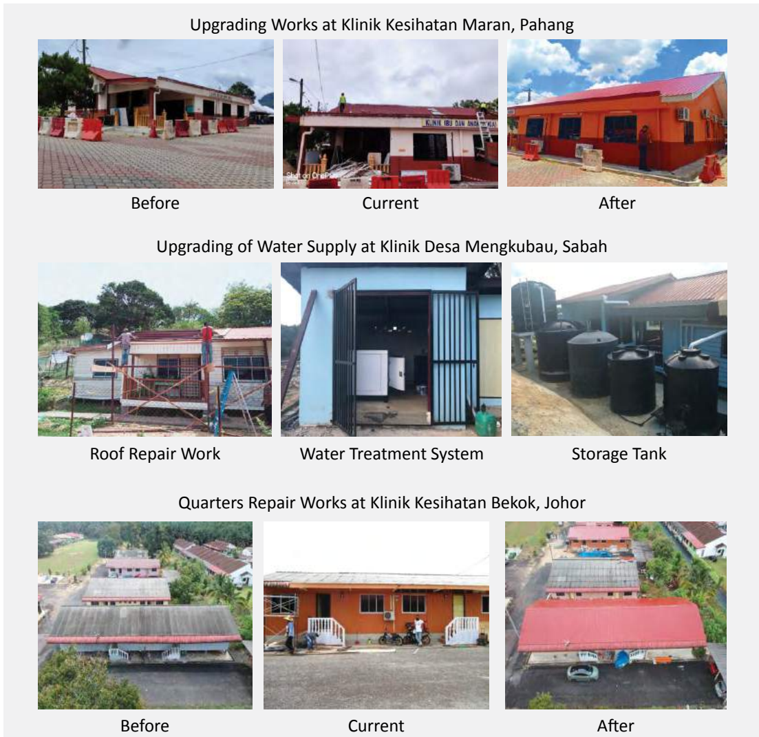
Image 6.23 Repair and Upgrading Works Building, Engineering Systems and Infra MOH Health Facilities in 2021
